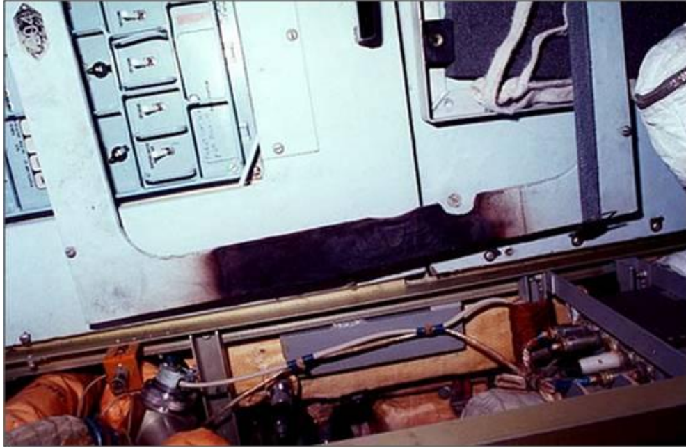
Figure 3: Fire-damaged panel onboard Mir, Credit: NASA.
